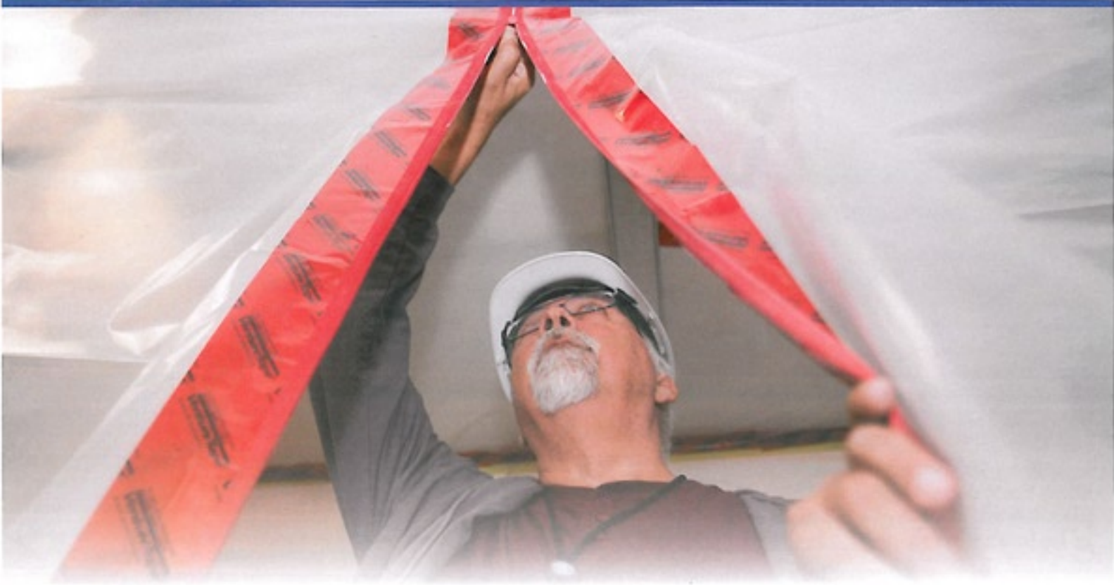
Bondfield Construction's senior site superintendent Bill Verhoog secures protective hoarding on 2 Shuter. Inside the plastic hoarding, a negative air machine runs to contain mold, dust and other particles within the construction zone. (Photo by Katie Cooper, Medical Media Centre)
